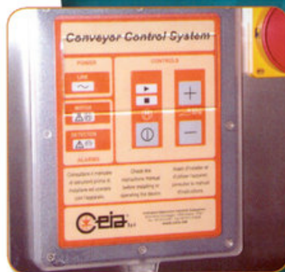
CONTROL PANEL ON CONVEYOR CONTROL SYSTEM
